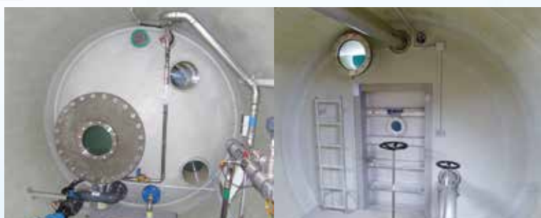
Access to water chamber
