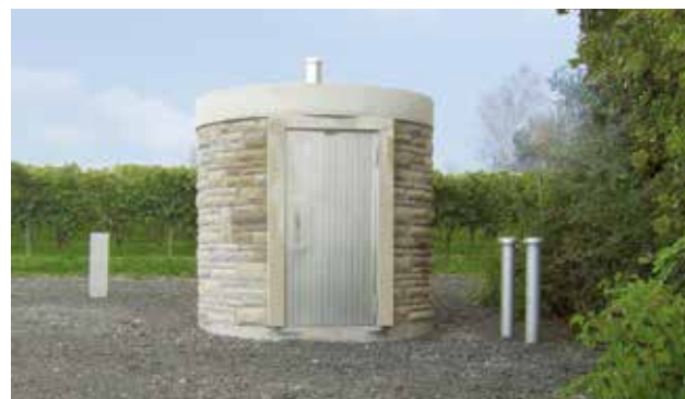
Water meter shaft
