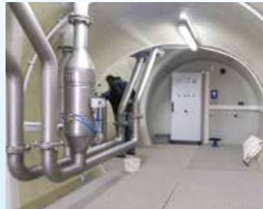
Pipework and fittings
