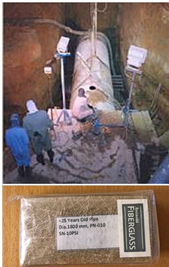
Fig. 9-10: A Flowtite GRP sewer pipe DN 1800 was unearthed and inspected after almost 25 years in service at a sewage treatment plant in Riyadh, SA. The pipe showed no signs of deterioration.
