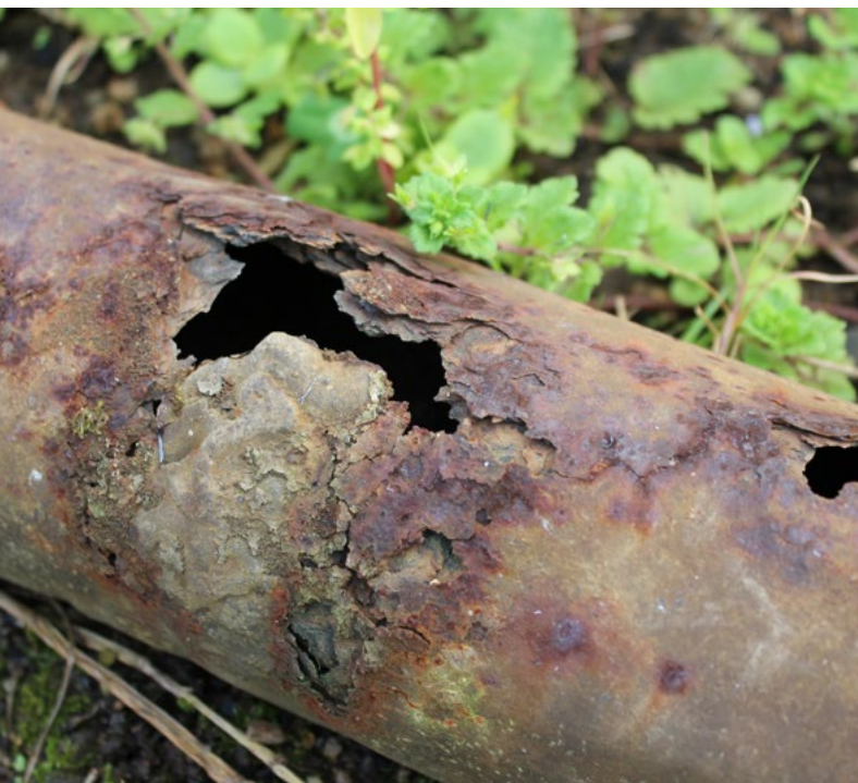
Fig. 1: Pipelines made of concrete or metals corrode in low-pH sewer environments under the influence of sulphuric acid.
