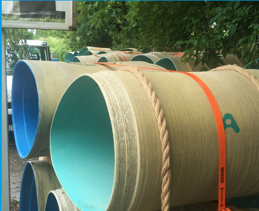
Above: 746 m of Amiblu NC Line pipes in various cross-sections were installed in the course of eight months to renovate parts of Krakow's aged sewer system.
