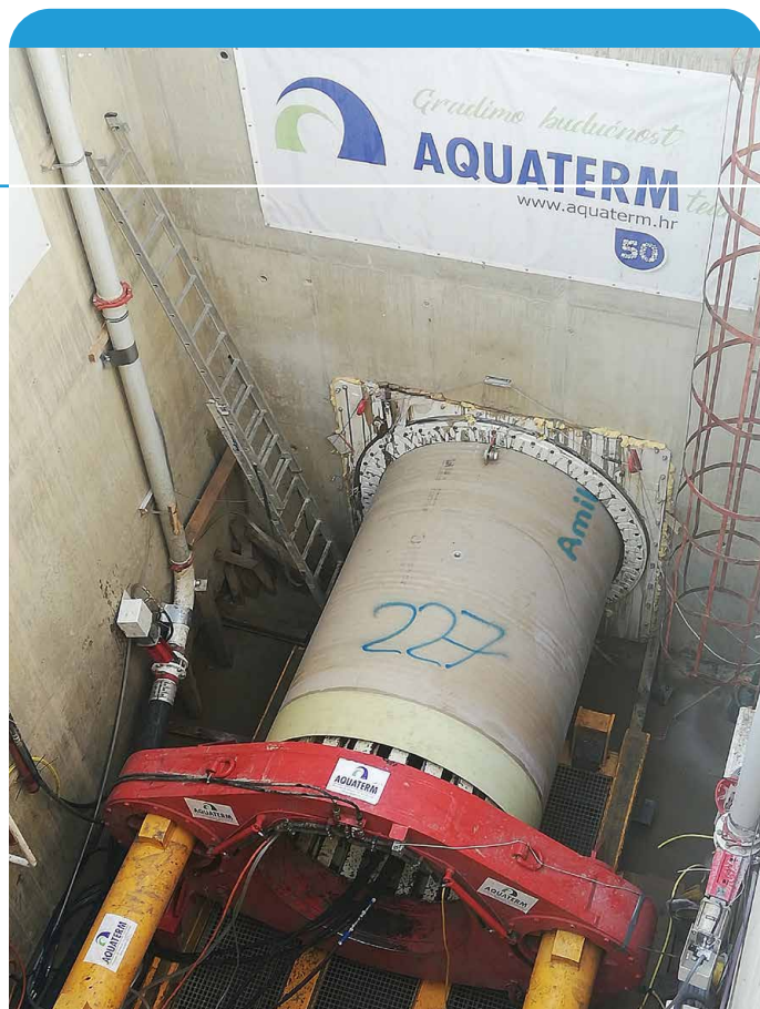
Amiblu CC-GRP pipes were jacked in a curve under the Sava riverbed with Herrenknecht equipment
