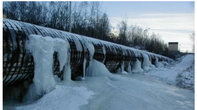
NO08HYL_Helleren 2 – Wooden penstock with severe leakage
