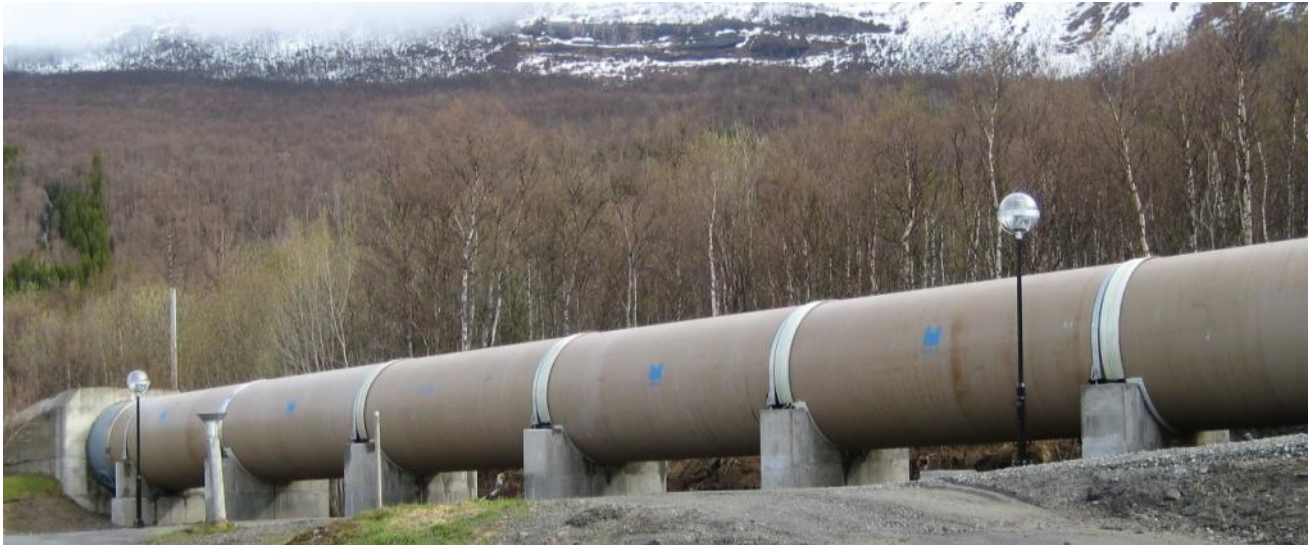
NO08HYL_Helleren 1- The new durable HOBAS Penstock DN 2500
